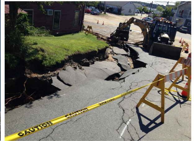
A giant hole appeared after heavy rains Wednesday night at Rufus Deering Lumber on Commercial Street in Portland. Yoon S. Byun/Staff Photographer
