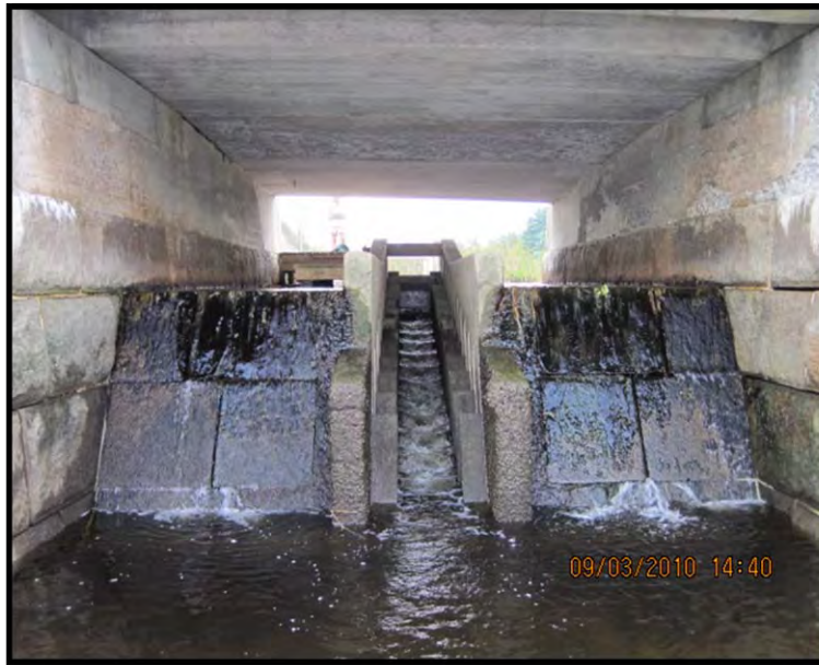
Winnegance Creek Dam with fish ladder, Phippsburg
